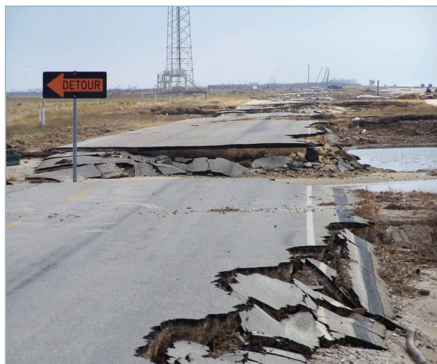
Figure 4. Ike's storm effects extended the destruction of Texas Highway 87 to the Bolivar Peninsula.
