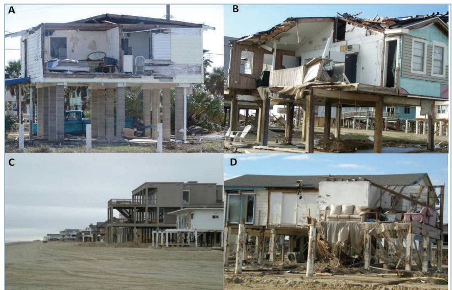
Figure 1. Damage caused by Hurricane Ike on Galveston Island. A. A house with its side ripped off. B. Destruction along the beach. C. A first row of houses was completely destroyed, leaving this second row as beachfront property. D. Remnants of a beach front house on the west end of Galveston Island.
